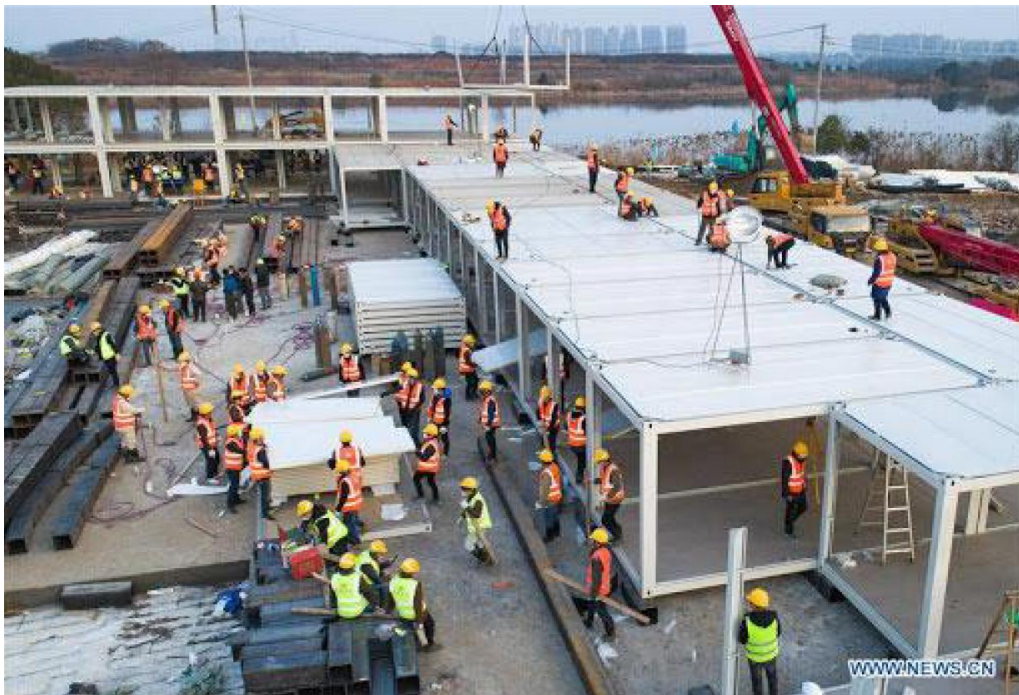
Image 16: Modular rooms being assembled during the construction of Covid-19 virus hospital in Hubei, China
